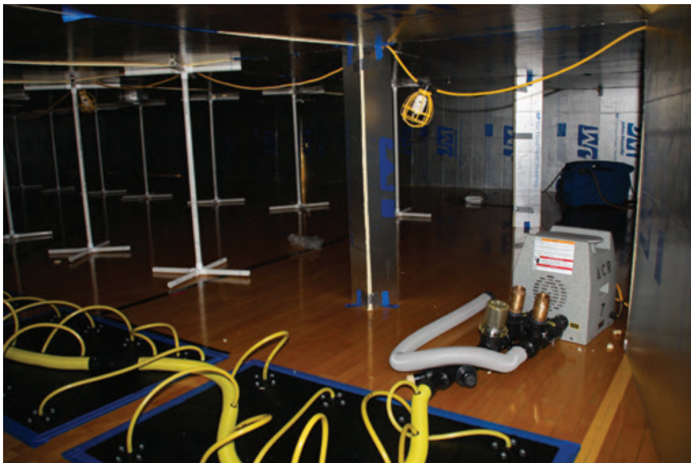
The set-up process required a highly coordinated effort by the entire response crew. Creating the temperature-control containment was a laborious undertaking. The process used all the restorative drying factors together, all under total technical control. Switchable lighting was added for additional safety in the confined space and to facilitate the meter-reading process.
